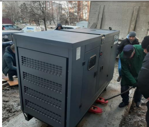
Salvation Church 25 KW Generator
